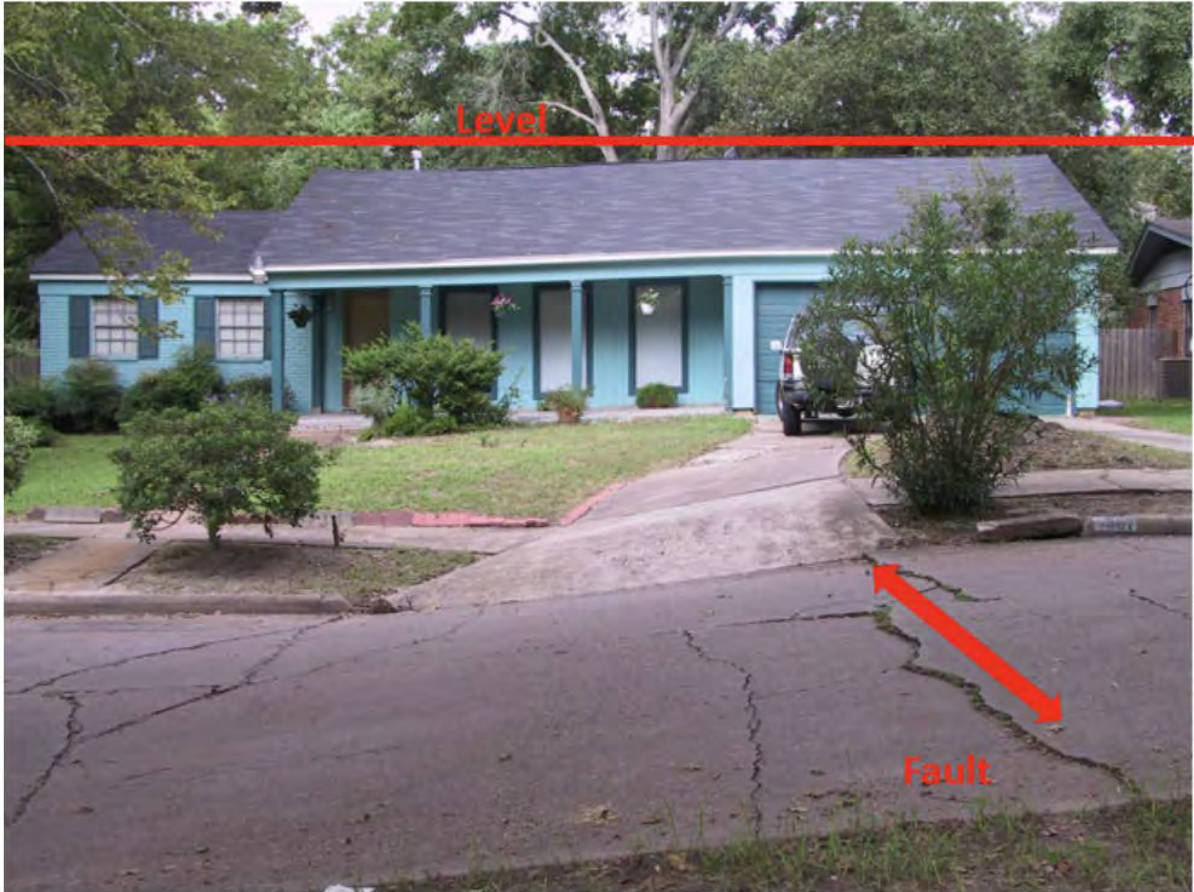
FIGURE 4-23. EXAMPLE OF FAULT IMPACTS ON A HOME IN GMA 14 (HOUSTON GEOLOGICAL SOCIETY, 2019)
