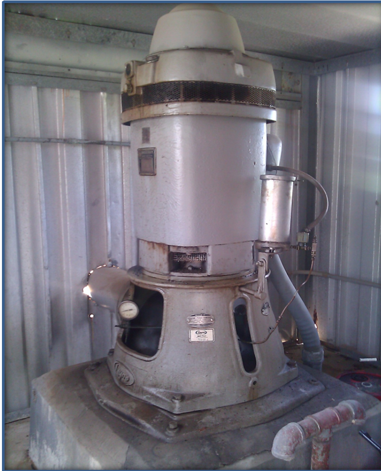
Figure 4: Well Pump at Station 21
