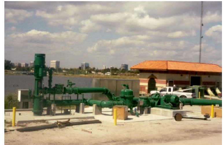
West Palm Beach, Florida ASR Well – 8 MGD Capacity Largest ASR Well in the World
