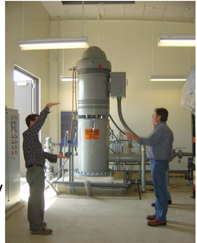
Calleguas MWD, California
